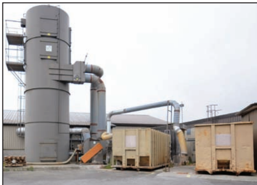
CONCEPT AIR 15 HP dust collector with (2) 60 HP discharge fans & rollaway dust bins
