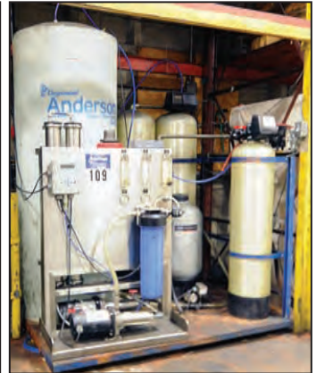
ANDERSON water treatment system
