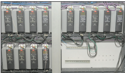
Partial view of VFDs available
