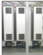
Partial view of VFDs available
