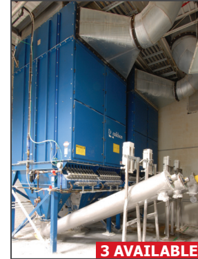
3 AVAILABLE View of DONALDSON TORIT DFT3-24 dust collectors
