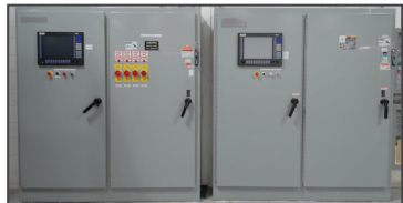
PLC controls for stainless steel product mixing system
