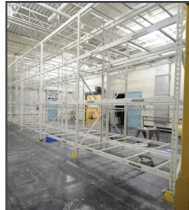
Partial view of rollout racking
