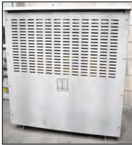
ELECTRICAL POWER INC. 225 KVA transformer
