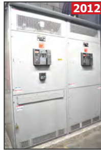
PIONEER FEDERAL twin bank switchgear unit
