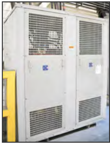
BEMAG 1250 KVA industrial transformer
