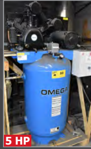
5 HP OMEGA air compressor
