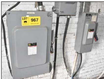
Partial view of SQUARE D electrical shut off switches available
