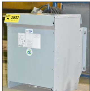
DELTA 45 KVA transformer
