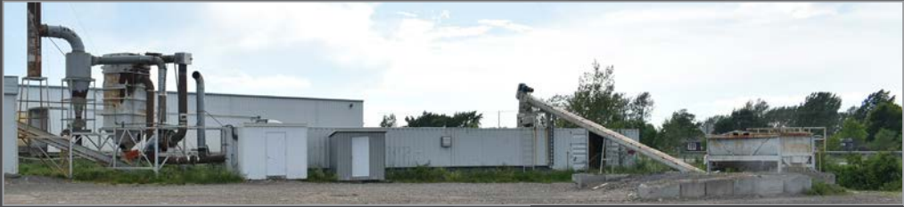
Custom mfg natural gas fired chip/dust dryer
